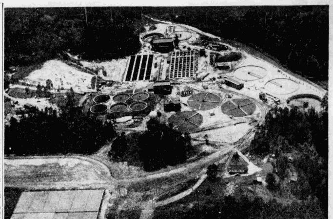
Aerial Photo Shows Progress Of Disposal Plant Construction (News Staff Photo by Tom Franklin-Franconi)
