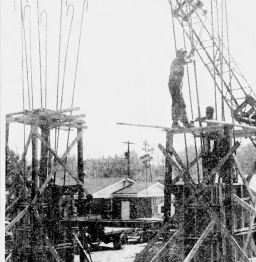
Supports for Highway 29 Bypass bridge going up in Beechwood Rd. back yards.
