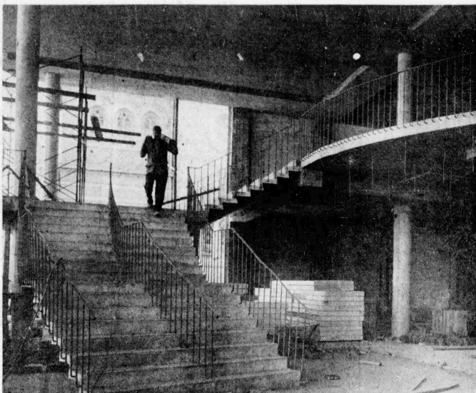
WITH THE WIDE STAIRCASE predominating, the interior of the new Charlotte Public Library is fast taking shape. The photo is the first made inside the building, being built on the site of the former library on N. Tryon St. The building, costing approximately $1 million, is due to be completed late this year. The library is now housed in temporary quarters on N. College St.
