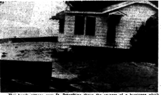
This beach cottage near St. Petersburg shows the ravages of a hurricane which moved through the Gulf of Mexico and struck inland Tuesday at Cedar Key, Fla. Pounded waves undermined the cottage and moved it several feet from its foundation. Waves continue to pound the bulkhead in the background. (AP Wirephoto).
