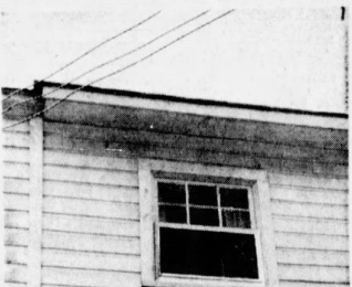
SUGAW CREEK DAMAGED THIS PARK RD. HOME The residence of David Cox stained by fumes in creek
