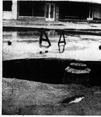
The culvert under the intersection of Dilworth Road and E. Morehead St. collapsed yesterday for the second time in recent weeks and the street caved in. The photograph was made shortly after a barricade had been placed
